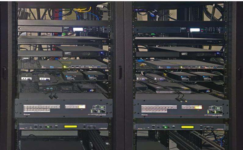
A centralized equipment room enables AV signal distribution to all points within the training center.
