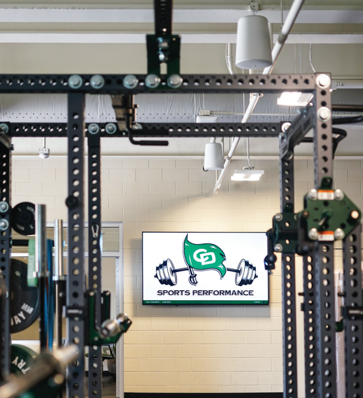
The weight room includes an 85" flat panel video display and a versatile sound system with wireless mics and SF 26PT SoundField pendant speakers over each weight station.
