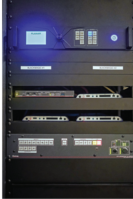
Gym AV equipment racks. Lefthand rack services the lobby; righthand rack services the sports court arena.
