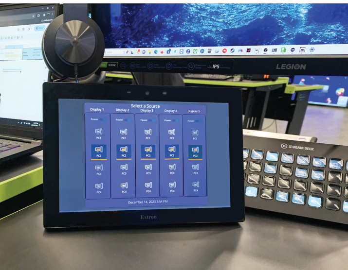
To manage the AV system, the operator uses the Extron TouchLink® Pro tabletop touchpanel at the production workstation.
