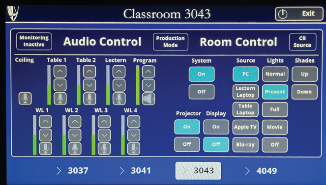
Touchpanels in all rooms feature intuitive buttons for setting all AV system functions and room lighting. (WL=Wireless, CR=Control Room).
