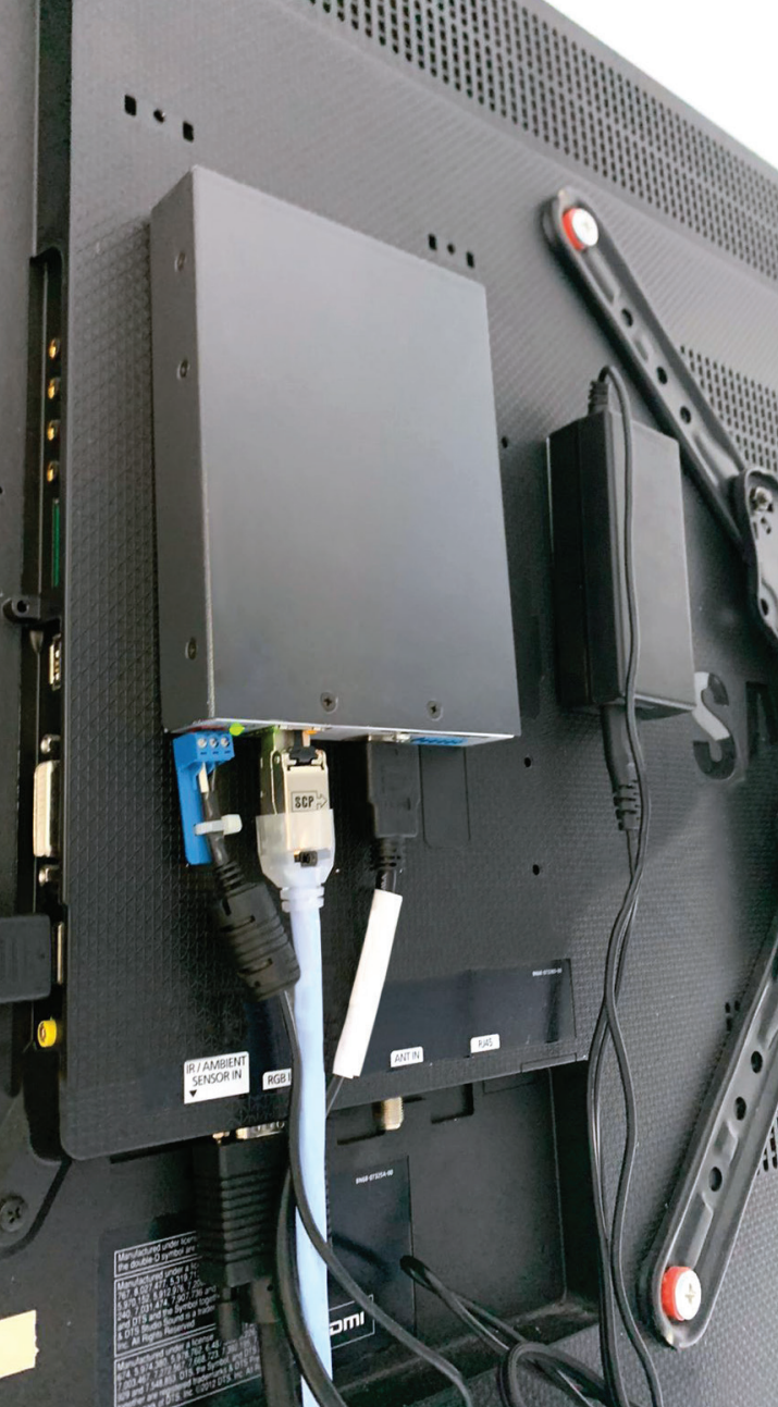
An Extron DTP 4K HDMI receiver is installed behind each display, receiving signals over twisted pair cable from the Quantum Ultra videowall processor in the equipment rack.
