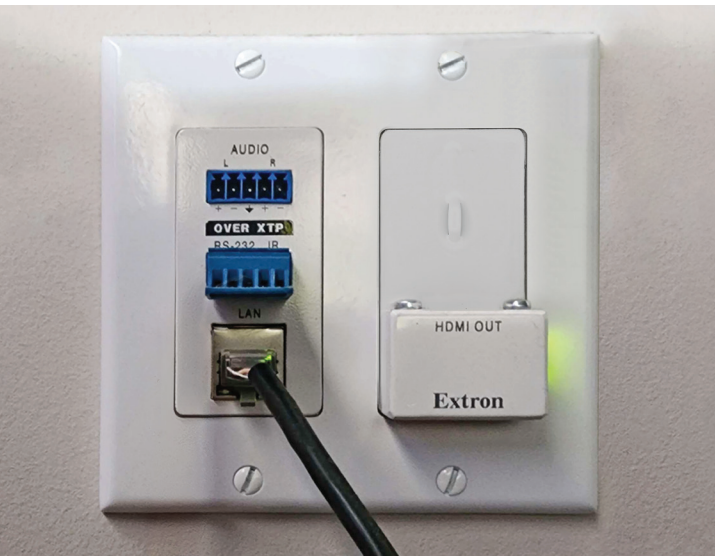
An XTP decorator-style wallplate receiver is installed behind each display, enabling a snug fit and clean appearance. For each projection system, an XTP scaling receiver delivers 4K HDMI video content at the projector's native resolution.
