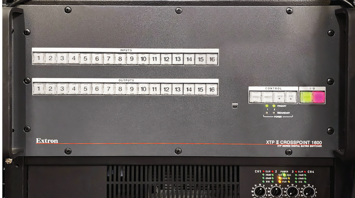
An Extron XTP II CrossPoint modular matrix switcher enables switching and distribution for AV and RS-232 control signals throughout the arena and its auxiliary locations.
