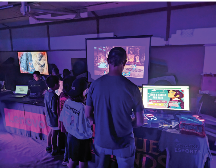
Projectors and large screen displays are mounted from the ceiling to enhance visibility without requiring valuable floor space. XTP receivers deliver 4K HDMI video content.
