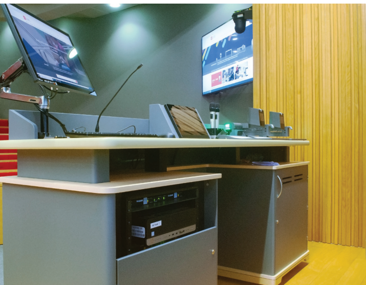
The presenter's table features an arm-mounted monitor, tabletop TouchLink Pro touchpanel, and built-in AV equipment racks for convenient, centralized control.
