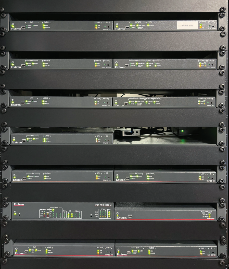
Left: The main control room rack houses Extron NAV endpoints and the NAVigator System Manager for efficient AV over IP distribution. Right: The compact but well-equipped control room integrates sound mixing and AV distribution within a streamlined, well-organized space.
