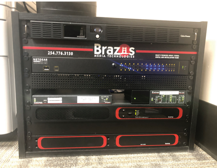
The compact sizes of the Extron NAVigator and IP Link Pro control processor allowed both units to fit easily into 1U of rack space.
