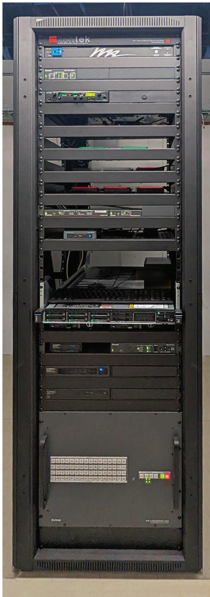
Equipment rack featuring Extron Pro Series Control and an XTP II CrossPoint 3200 modular matrix switcher with a 50 Gbps digital backplane, essential for maintaining smooth AV function.
