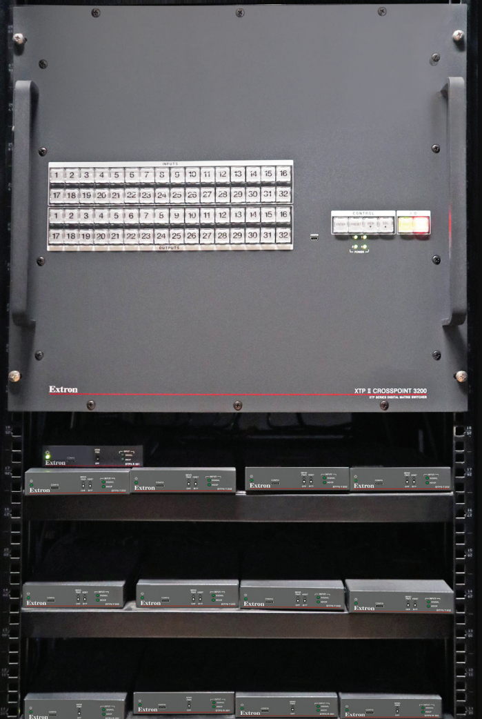
Extron XTP II CrossPoint 3200 modular digital matrix switchers along with DTP3 T 202 HDMI transmitters and DTP3 R 201 receivers deliver robust 4K/60 signal routing and reliable AV performance.
