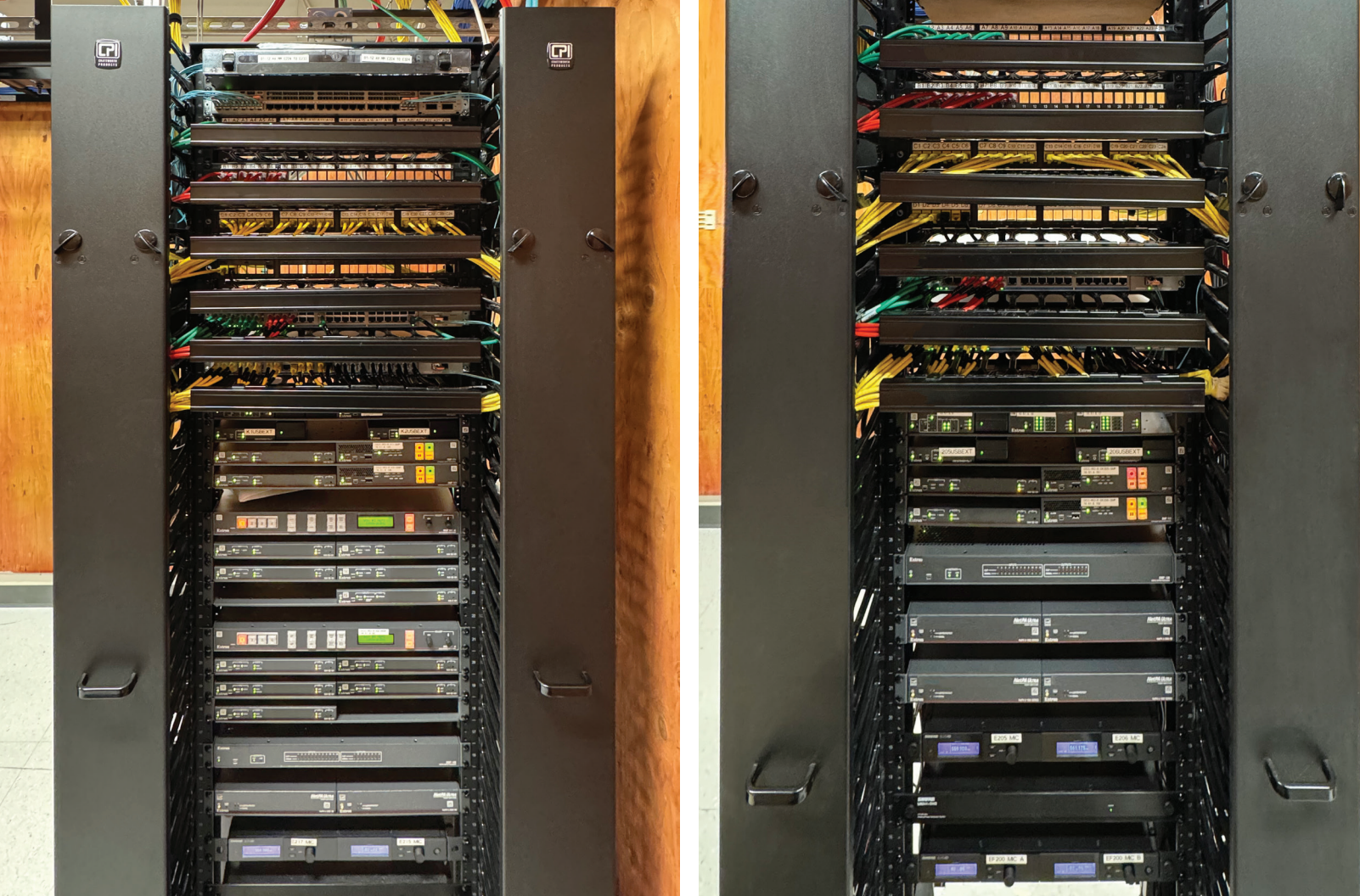
AV racks are located in telecommunications rooms on each floor of the building.
