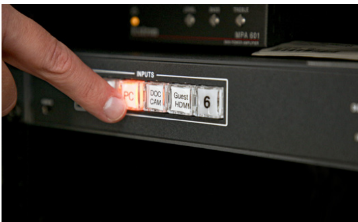
The switcher's clearly labeled buttons that light when pressed make AV source selection easy. Buttons 1 and 6 are spare inputs that allow future expansion.
