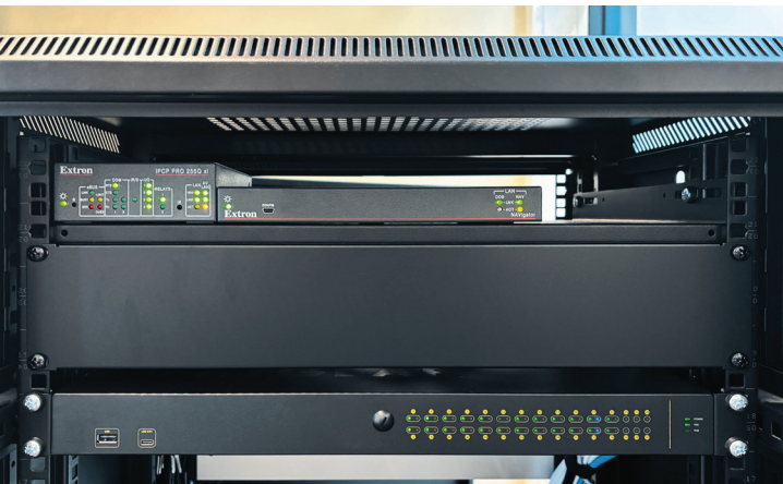
The equipment rack houses the Extron NAVigator System Manager, IPCP Pro 255Q xi control processor, and Netgear AV Line switch, forming the backbone of each classroom's AV network.
