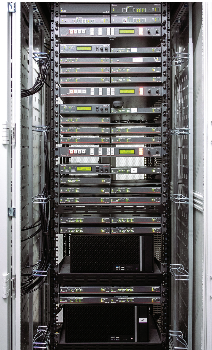
The Extron NAV Pro AV over IP System enables signal switching and distribution from a central location and is essential for maintaining smooth AV functions throughout the Echo building.
