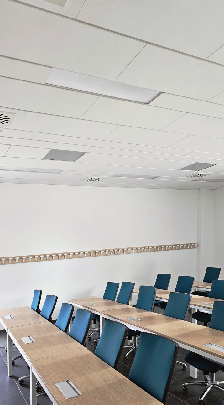
Extron FF 220T ceiling speakers provide a very wide room coverage pattern throughout the library.
