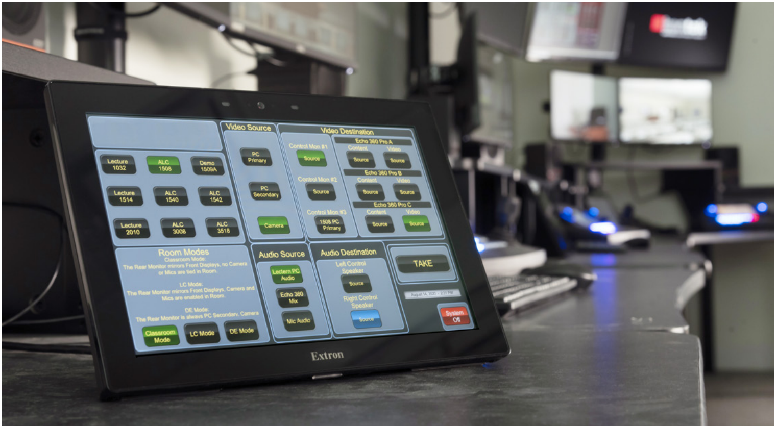
The primary user interface in the Control Room allows the operator to easily monitor and assist an instructor in any room.
