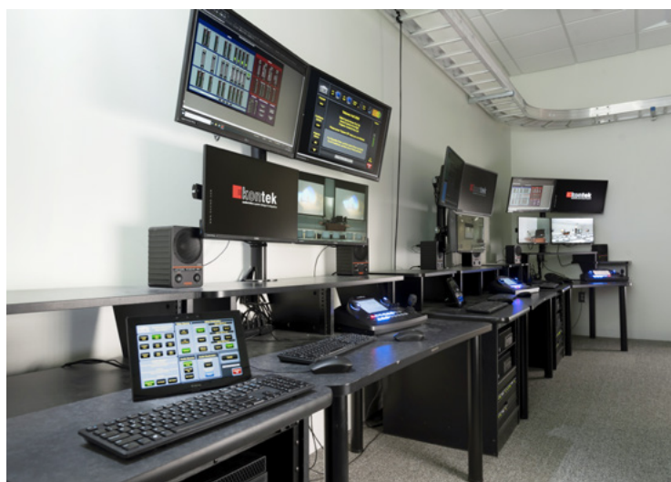
Veterans Hall Control Room with three stations for monitoring multiple classrooms simultaneously.
