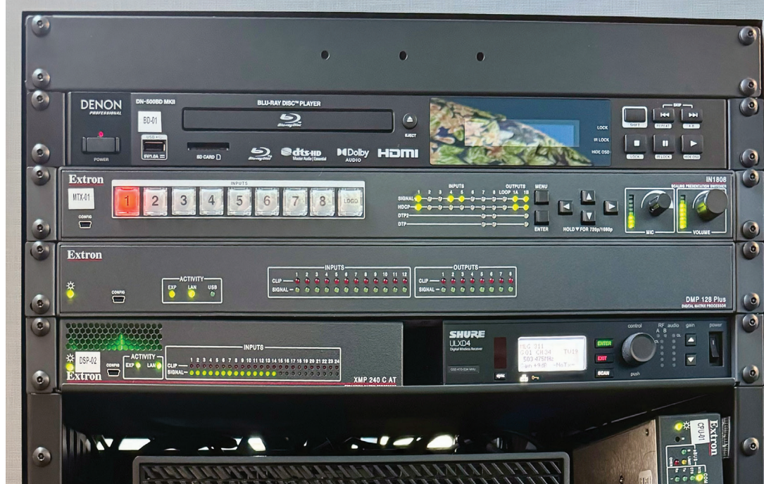
Detail view of Extron equipment in classrooms 301 and 311 AV equipment racks.
