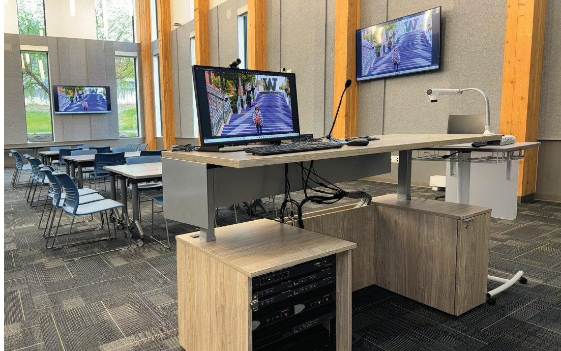
HIPs adjustable-height lectern with AV equipment bay housed in lower left cabinet enclosure.
