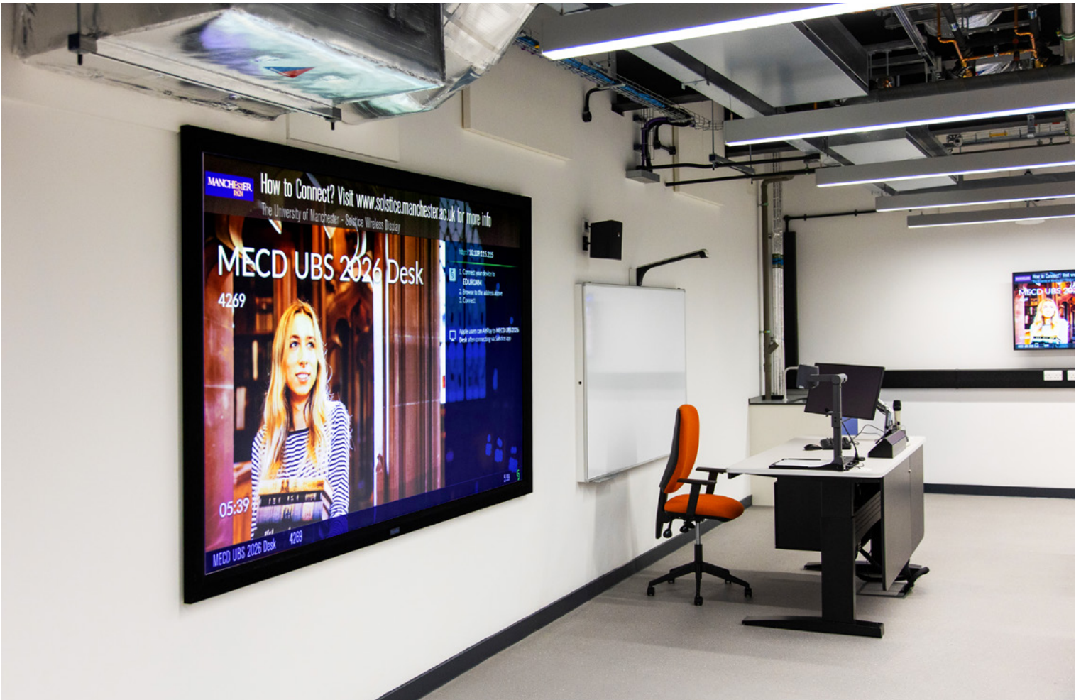
The small Meet & Teach rooms provide at least one display and an AV system based on an Extron SW HD 4K PLUS 4K/60 HDMI switcher. Intuitive AV system control is provided by an Extron TouchLink Pro touchpanel or Network Button Panel.
