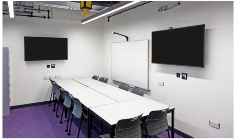
Student spaces provide access to the same resources as classrooms. An Extron MediaLink controller and a network button panel enable source selection and local display control.
