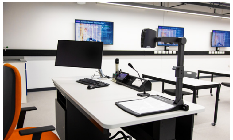
Using the Extron TouchLink Pro touchpanel at the AV-enabled lectern, the instructor can switch sources to present the same content on all displays, enable each group to control their local display, or share content sourced from a workstation or another room.
